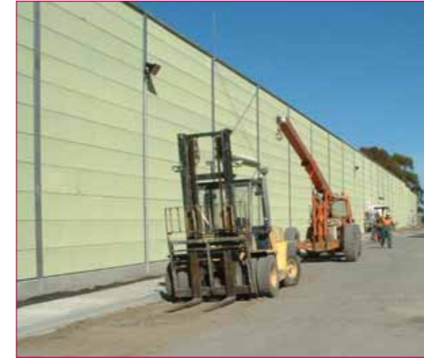
Whirinaki Power Station
